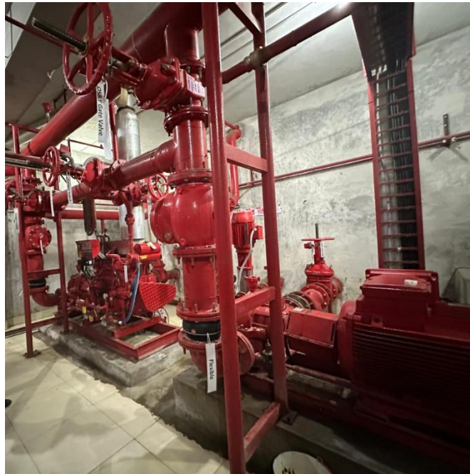
Figure 10: Underground Fire Safety Pump.
